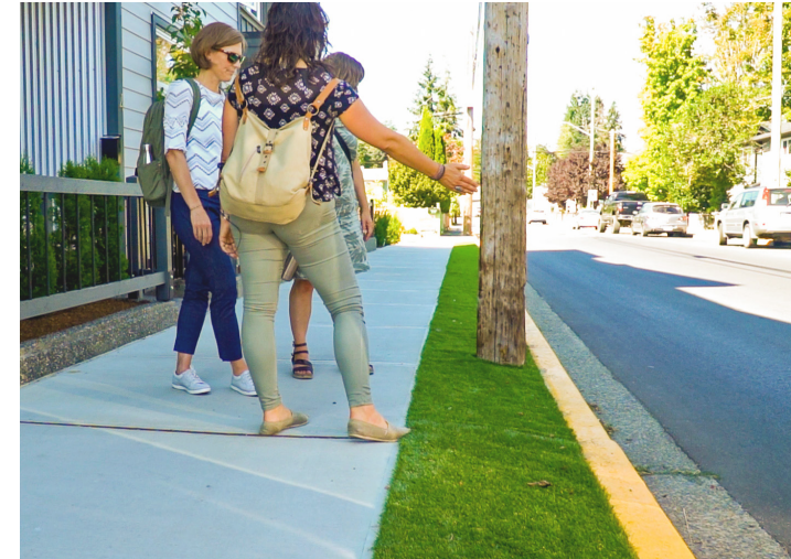
Artificial turf beside the new sidewalk on Jubilee Street acts as a temporary, cost-effective measure to protect space for the upcoming bike lane installation.
