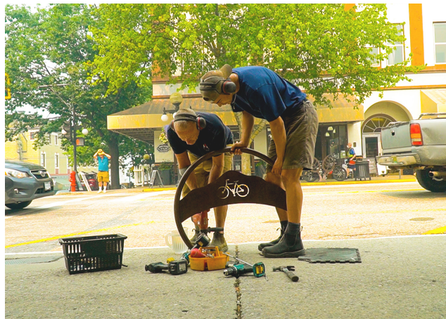
Workers install a bike rack on the sidewalk, next to downtown street parking. This encourages people to cycle throughout the downtown core.
