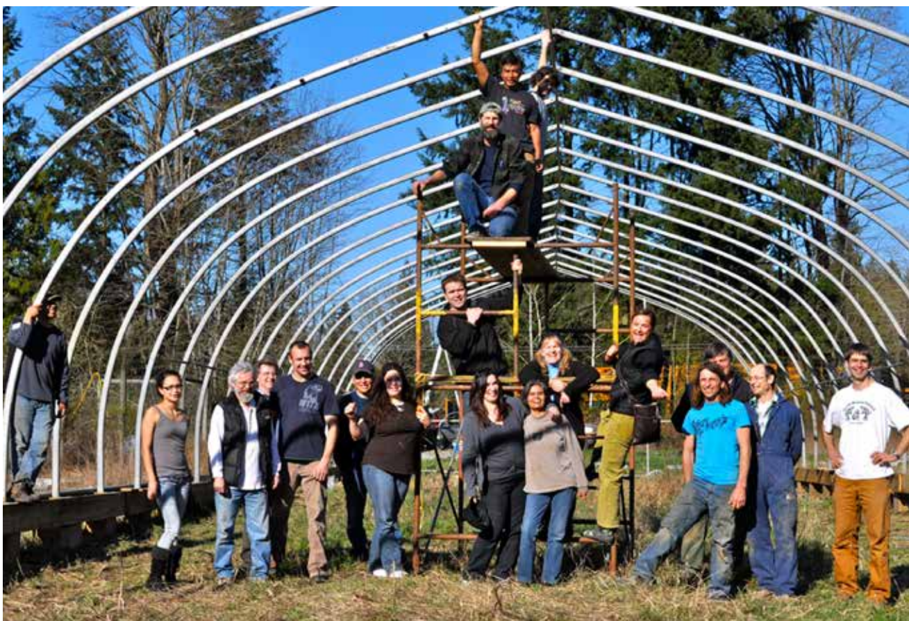
Greenhouse in Delta is built with support from BCHLA's Community Capacity Building Initiative
